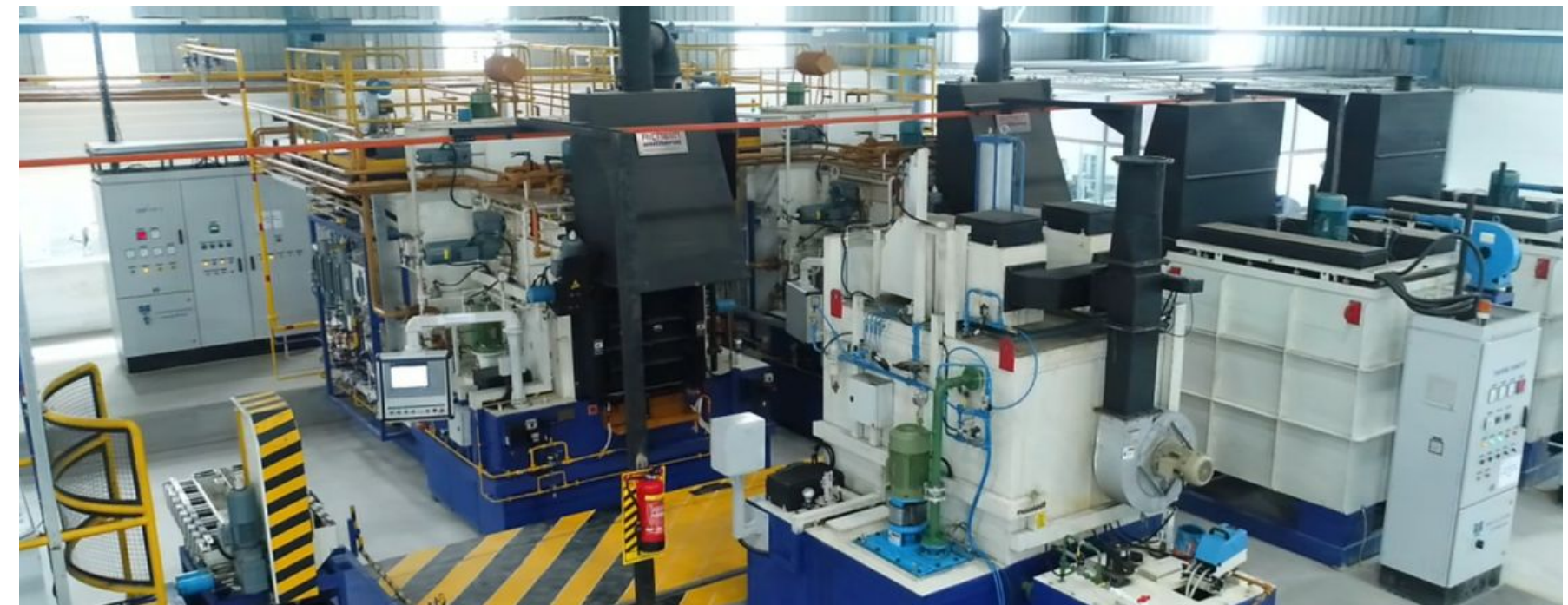
Sealed Quenched Furnace(2) | Aichelin Unitherm
